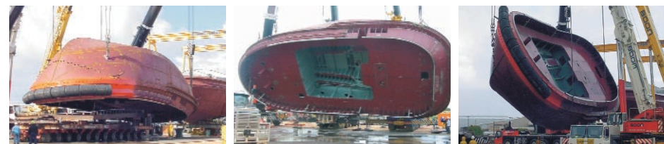
Lift, roll and lower ... the progressive moves to roll over the hull of a new tugboat built in W.A
