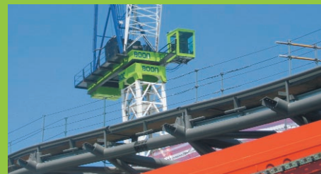
Looking over the Melbourne CBD city skyline and more of the many BOOM cranes are appearing in green.
