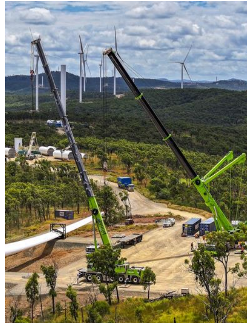
Clarke Creek Wind Farm Northern QLD Turbine construction project 250t & 500t All Terrains
