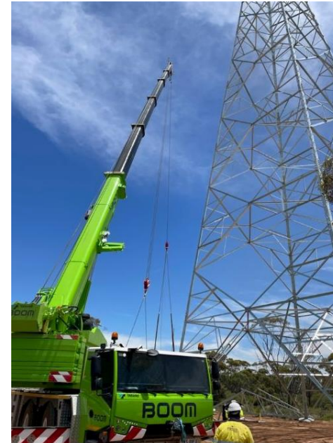
Energy Connect Transmission Project NSW 700km SA to Wagga Wagga Cranes 60t to 150t
